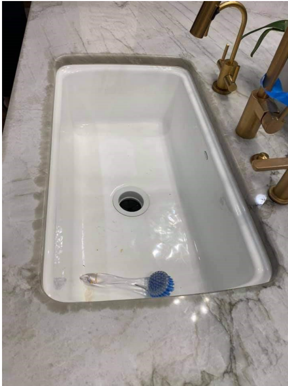
Fig. 2: Stain pattern at the cut surfaces in the sink area
